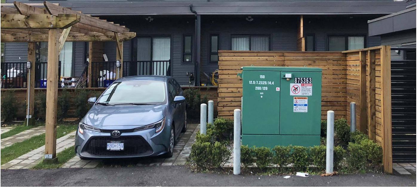
Pad mounted transformer. Credit: City of Vancouver
