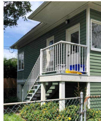
Figure 7. Landing in rear yard
